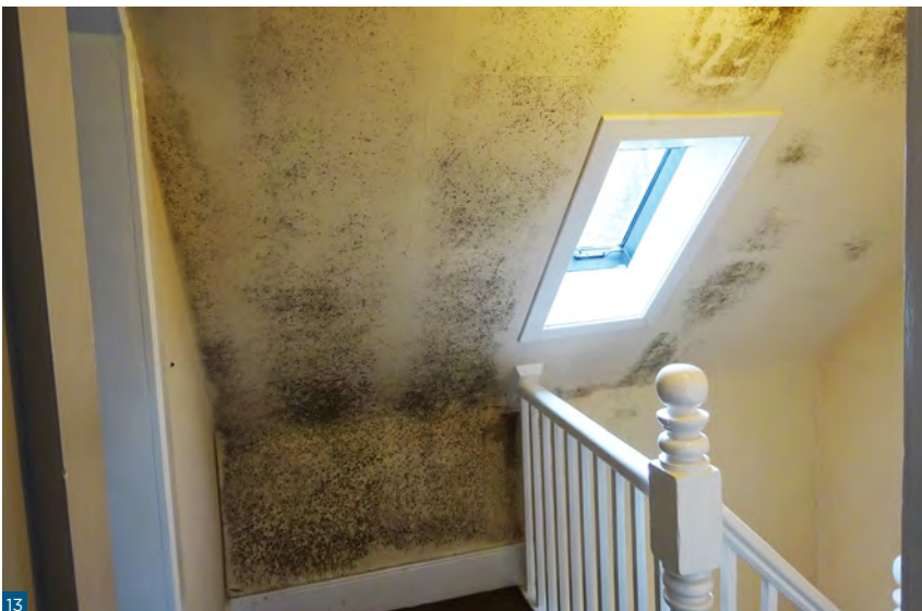
Figure 13: Vapour impermeable materials and a lack of ventilation have led to significant mould growth on internal surfaces in this building.
