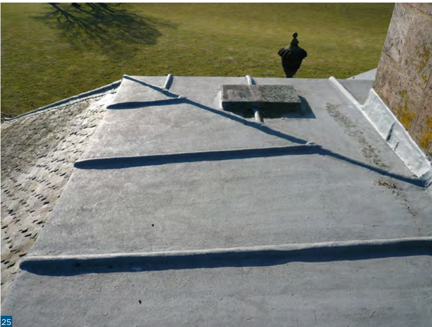
Figure 25: Care is required where a flat roof is covered in lead or other metal not to cause conditions on the underside that lead to corrosion following retrofit.
