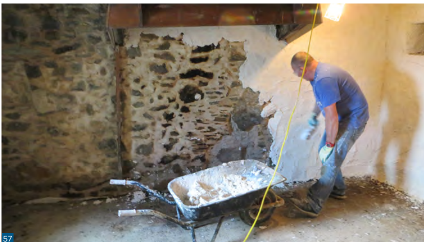
Figure 57: First coat of insulated lime plaster being applied directly to the masonry of the Category A-listed Downie's Cottage, near Braemar. A second coat is applied in much the same way.
