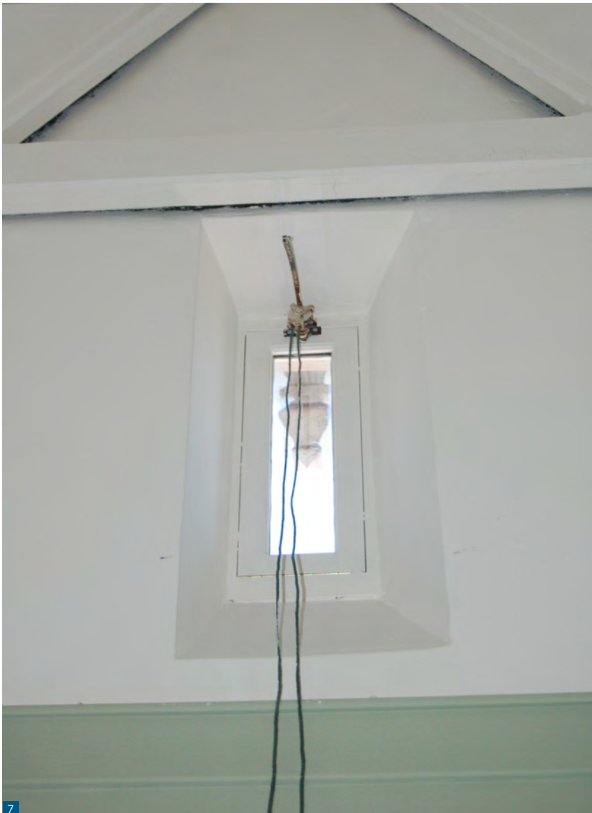
Figure 7: This quarter light has been made to open to allow managed ventilation.
