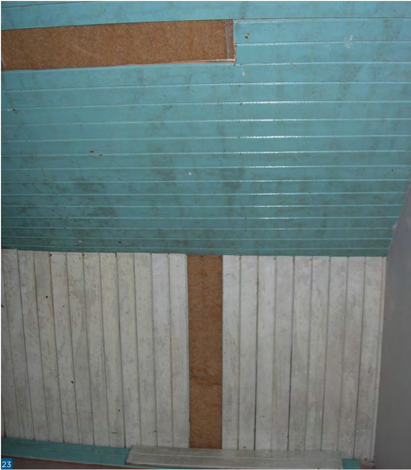
Figure 23: Wood fibre board used behind an existing timber lining on a coom.
