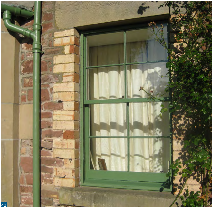
Figure 42: External secondary glazing which gives weathering protection, as well as a degree of thermal improvement.
