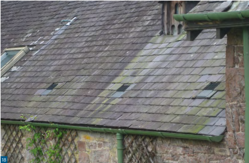
Figure 18: Low profile roof vents on a slate roof following an upgrade to the roof space.
