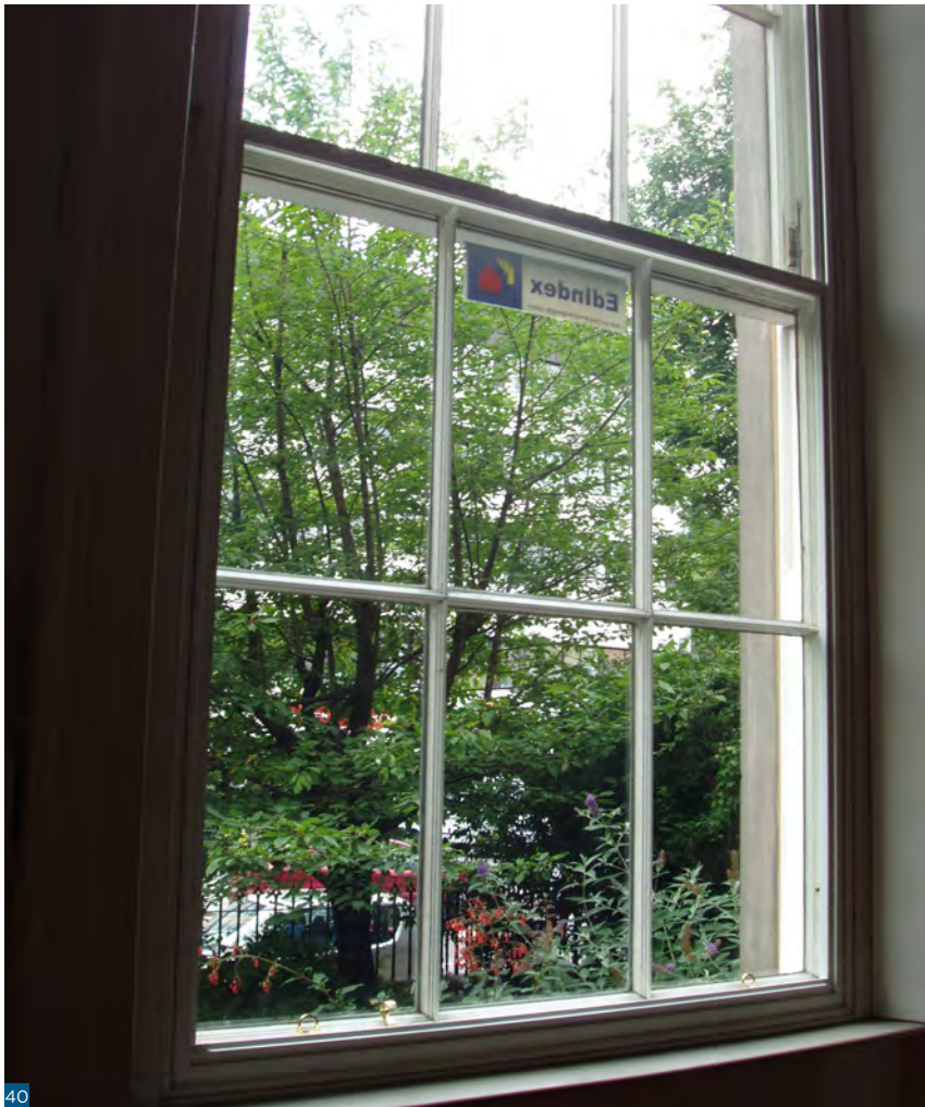
Figure 40: Secondary glazing mounted within the staff beads, allowing the use of shutters.
