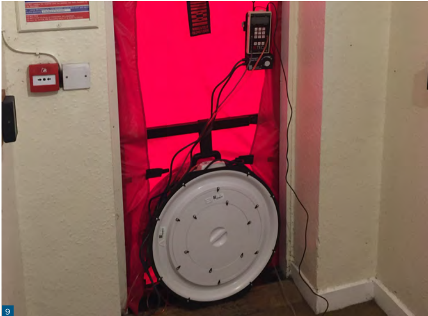
Figure 9: An air pressure test taking place at Holyrood Park Lodge before the interventions.
