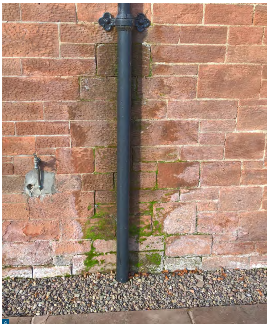
Figure 4: All buildings should be well maintained, and any defects should be repaired before any retrofit work is undertaken. This downpipe has been blocked for some time and the masonry behind appears to be saturated; this defect should be addressed first before any insulation work.
