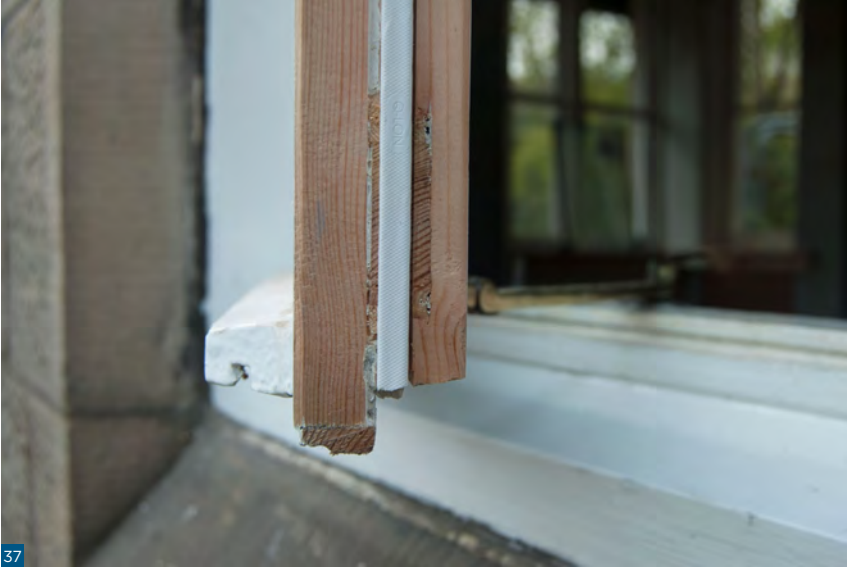
Figure 37: A newly fitted brush strip (white) on a casement window at Holyrood Park Lodge.
