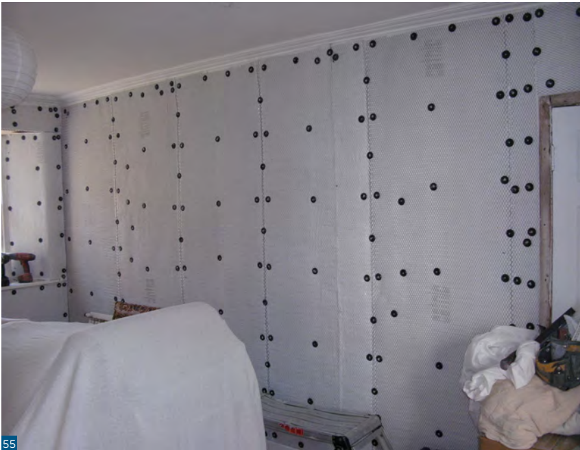
Figure 55: Aerogel blanket applied directly to masonry using thermally decoupled expansion fasteners ( Refurbishment Case Study 3 ).
