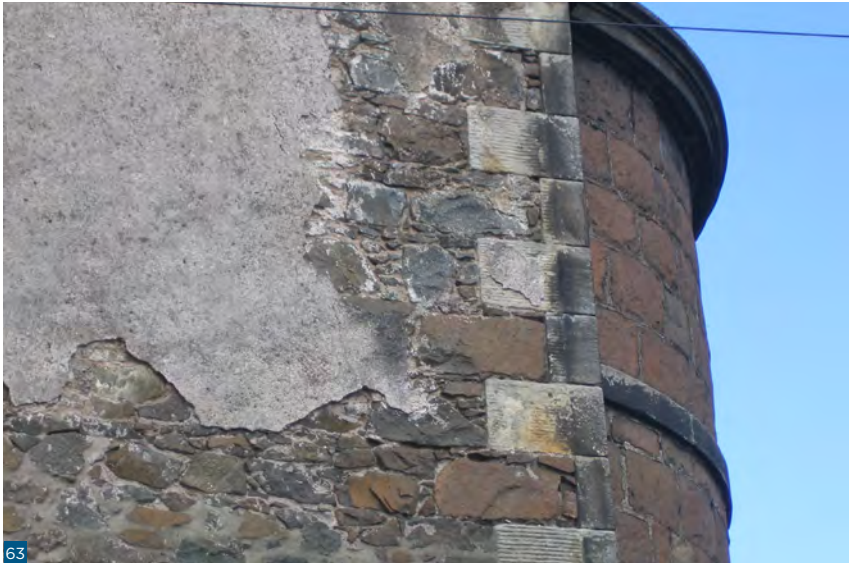
Figure 63: This gable end, which is in need of maintenance and showing the remains of a lime render, is well placed to receive an appropriate form of thin external insulation.
