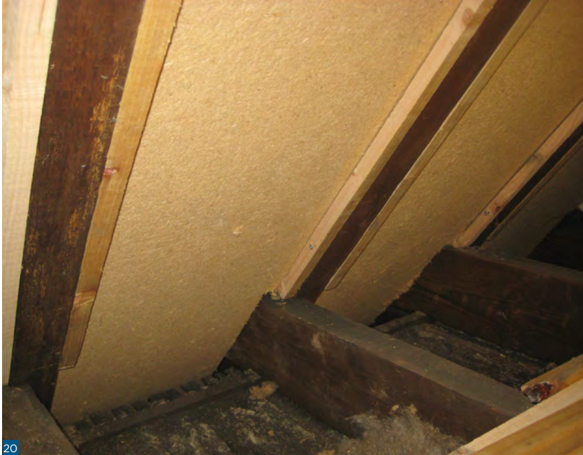
Figure 20: A roof slope insulated with a wood fibreboard insulation between the rafters.
